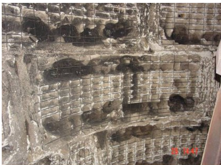
Figure 35: Damage suffered by the tunnel lining at the level of the tunnel roof
