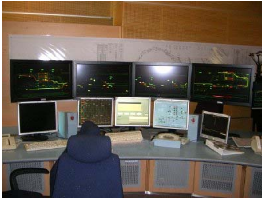
Figure 15: Rail traffic management (RTM) controller's workstation at the RCC on the French side
